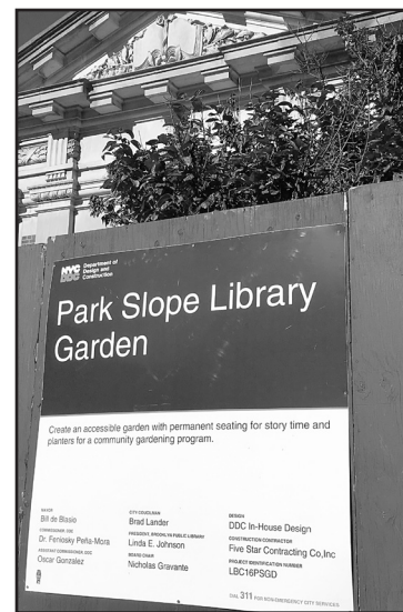
At the Park Slope Library (at Ninth St. and Sixth Ave.), the City is constructing a child-friendly amphitheater for outdoor storytelling.
